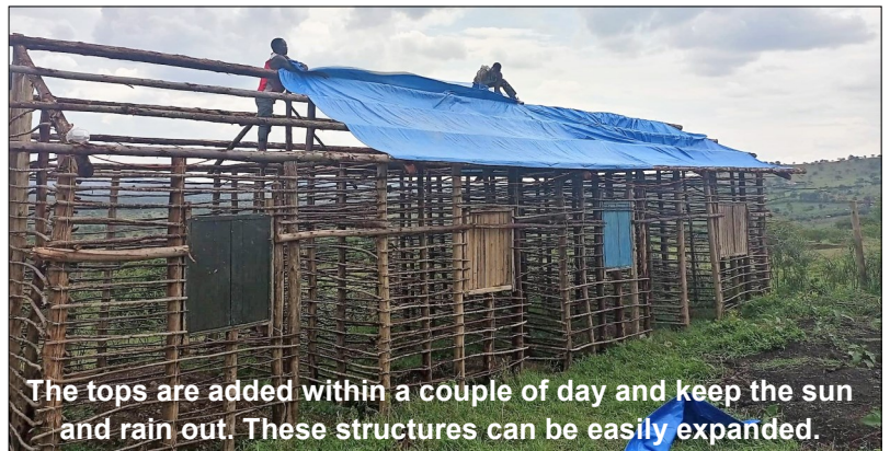
The WAY Community Churches initial pole structure is put up in a days time with 30 men working together.
