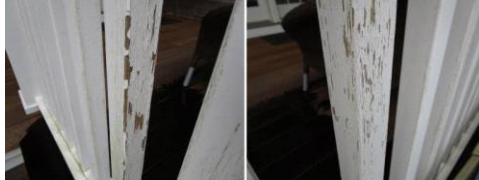
minor peeling on guardrails
