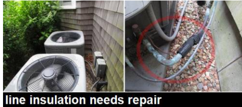
line insulation needs repair
