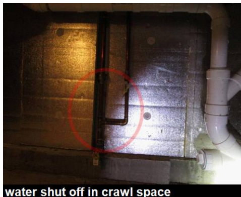
water shut off in crawl space
