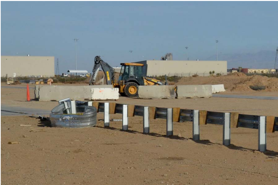
FIGURE 26. Post-Test Left Rear \frac{3}{4} View of Test Article
