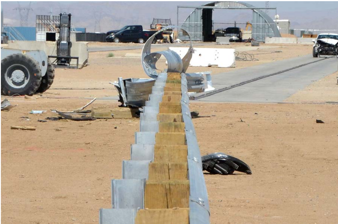
FIGURE 24. Post-Test Rear View of Test Article
