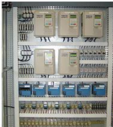
AC Drive Panel
