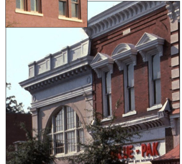
Windows add not only light, but interest. Note the various types of trim and moldings on the cornices and windows of these buildings
