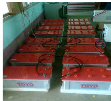
Fig. 6 200Ah batteries for storing the charges for later use.
