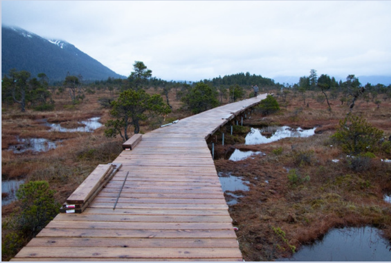
The Mountain View Manor boardwalk construction began in September; 20% of the boardwalk has been completed.
