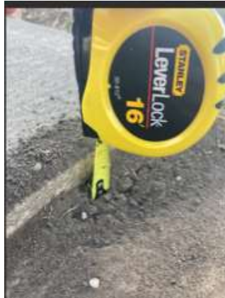
Figure 4. Trip hazard: 2 inch sidewalk crack
