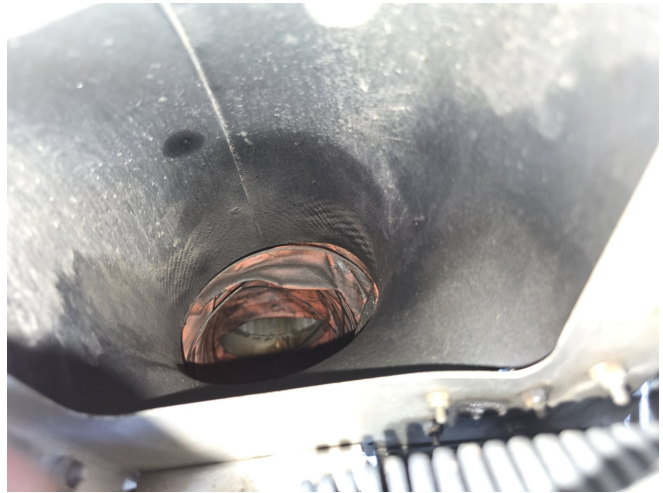
Figure 4 - Collapsed Oil-Cooler SCAT Hose at Cowling Connection The view through the cowling connection confirms that the oil-cooler cooling-air hose is collapsed and substantially restricted. This condition reduces airflow through the oil cooler and likely contributed to the reported high oil temperature.
