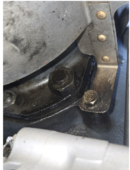
Figure 10 - No. 1 Cylinder Underside Oil Leak The underside of Cylinder No. 1 and the adjacent crankcase and attachment area exhibit heavy oil saturation and accumulated residue consistent with a longstanding, unresolved leak. Oil migrating downward from this area has contributed to the extensive contamination and heat-baked deposits observed on the muffler shroud below.
