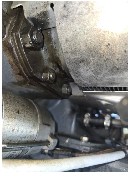
Figure 9 - No. 2 Cylinder Base and Hold-Down Nut Oil Leaks After the engine was cleaned, operated, and reinspected, oil leakage was confirmed at the base area of Cylinder No. 2. Oil leaking through the upper cylinder hold-down nut is also contributing to the extensive saturation of the cylinder, adjacent crankcase, and surrounding components. The amount of contamination is consistent with longstanding, unresolved leakage.
