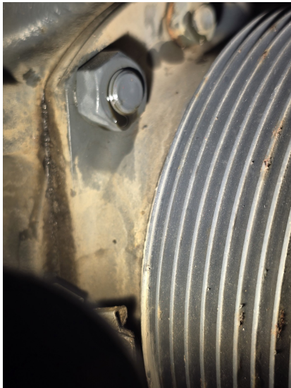
Figure 7 - No. 2 Cylinder Hold-Down Nut Oil Leak Fresh oil is visible around the No. 2 cylinder hold-down nut. This leak contributes to the same longstanding oil saturation documented at the No. 2 cylinder base, adjacent engine area, and muffler shroud. The attachment hardware, stud, crankcase area, and sealing surfaces require further inspection.
