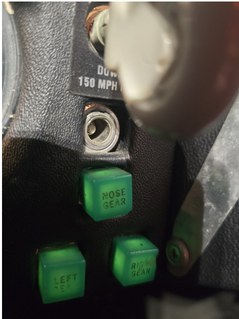
Figure 6 - Missing Gear Unsafe Warning Light and Housing The landing-gear unsafe-warning-light lens and housing are absent, leaving the receptacle opening exposed. The three green individual gear-position indicators remain installed below it.
