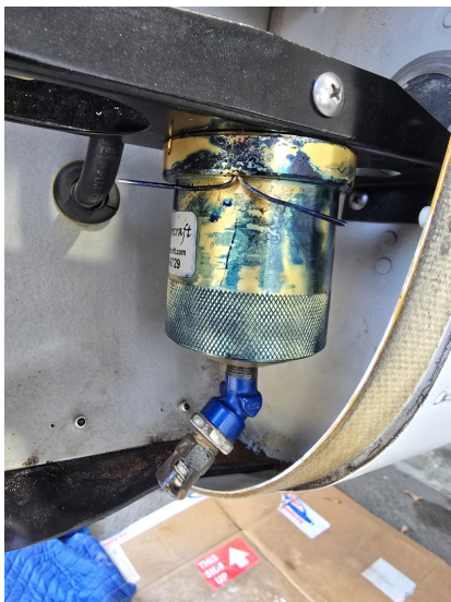
Figure 5 - Fuel Staining at Gascolator Significant blue fuel staining is present on the gascolator bowl and around its upper seam, indicating a current or previous fuel leak. The assembly requires inspection and leak testing.
