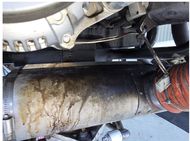
Figure 8 - Oil Contamination and Heat-Baked Deposits on Muffler Shroud The muffler shroud exhibits extensive oil staining and heat-baked deposits directly below Cylinders Nos. 1 and 2. The accumulated and burned-on residue is consistent with prolonged exposure from the unresolved oil leaks at those cylinders rather than a recent isolated event. Oil contacting the hot exhaust and muffler assemblies presents a potential smoke and fire hazard.
