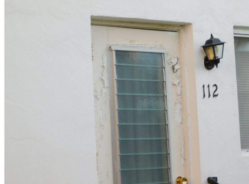
Unprotected Glazed Entry Door
