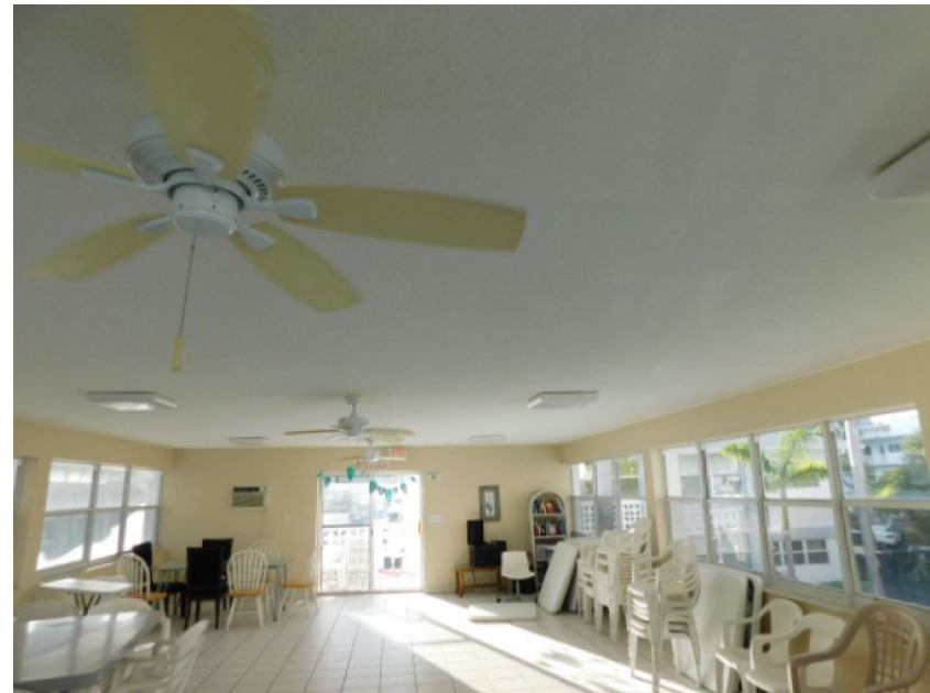
No Attic Access
