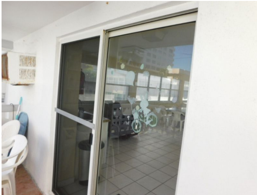
Unprotected Glazed Entry Door
