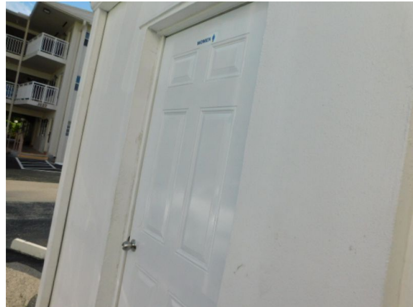
Unprotected Solid Entry Door
