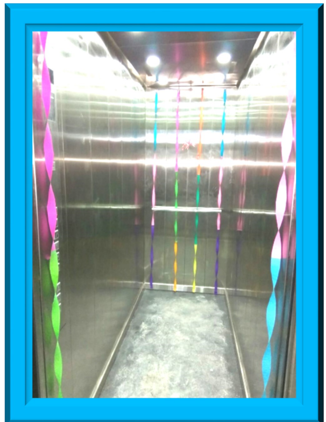
Newly Installed Elevator
