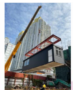
Cargo Lifting Monitoring
