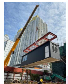
Cargo Lifting Monitoring
