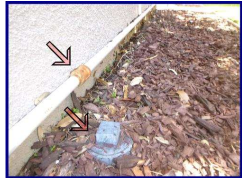
rust at gas pipe / unpainted cleanout
