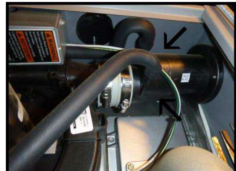
hose not clamped
