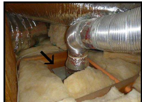
uninsulated top of register box here
