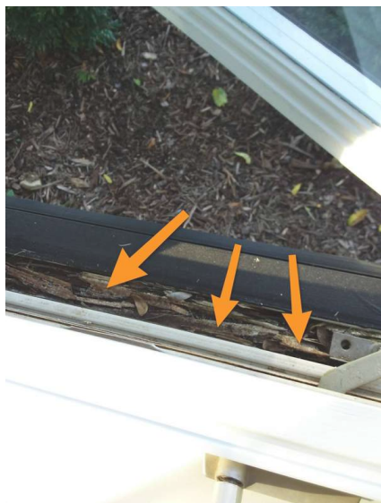
Rotted interior sill.
