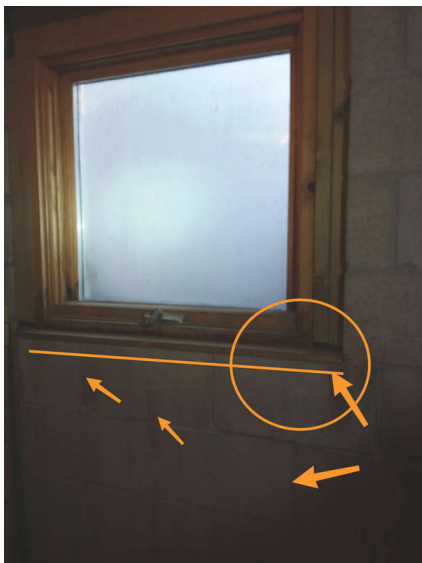
Water stains and moisture issues
