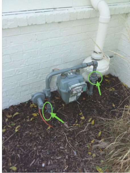
Main Gas Shut off
