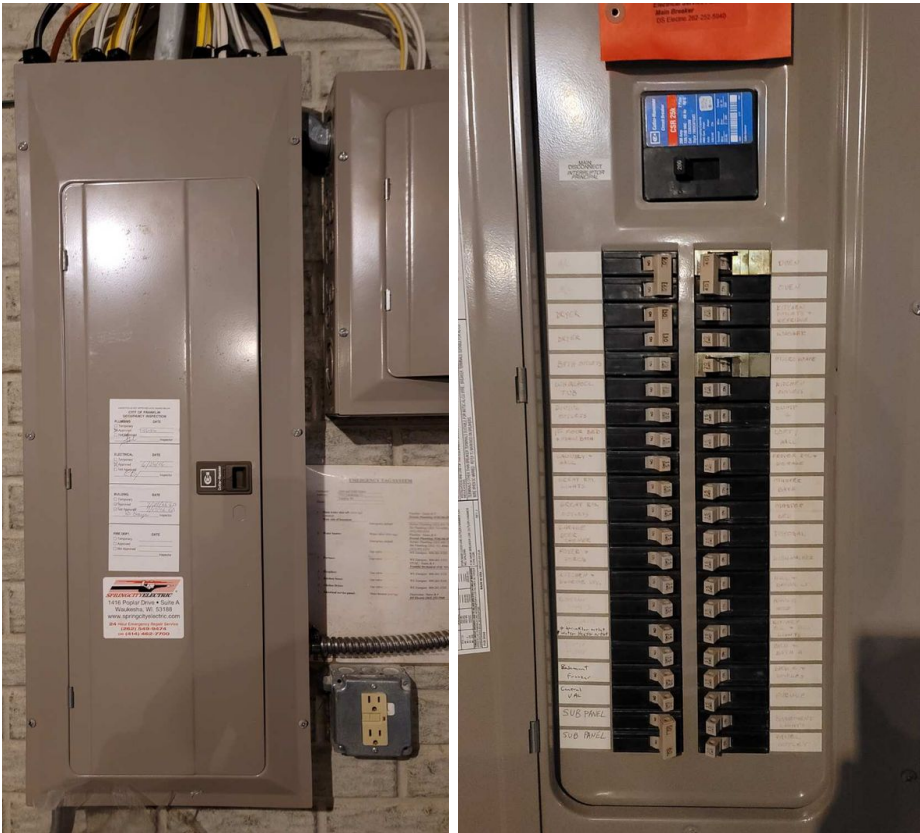
Main & Subpanels, Service & Grounding, Main Overcurrent Device: Panel Manufacturer Cutler Hammer
