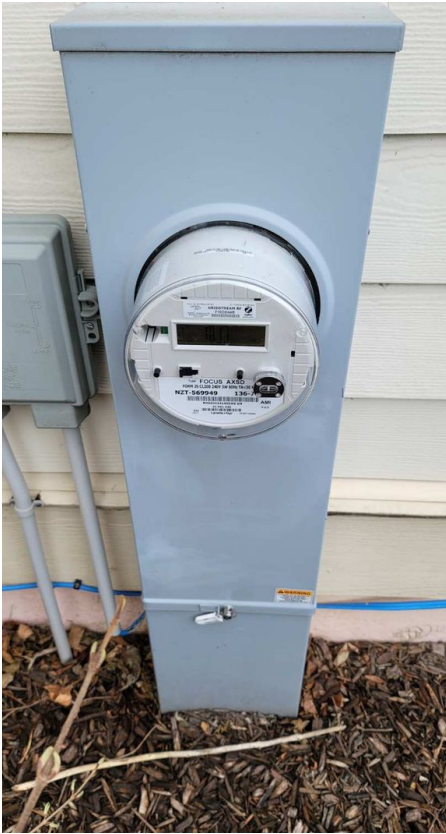
Main & Subpanels, Service & Grounding, Main Overcurrent Device: Panel Capacity 200 AMP
