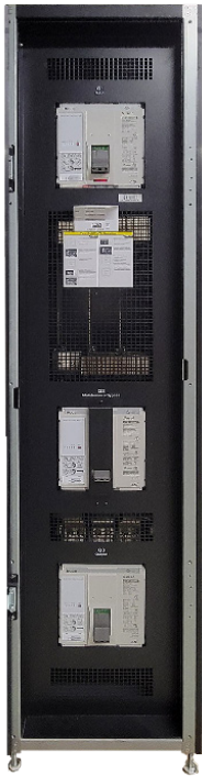
Maintenance bypass (door removed)
