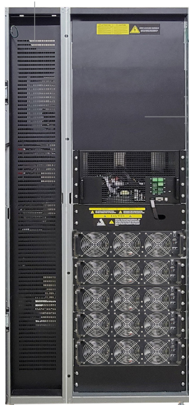
X90-5S 350kW UPS (door removed)
