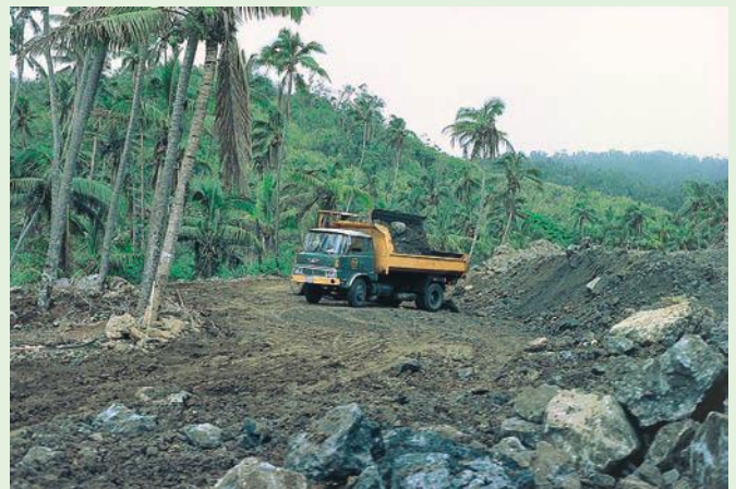
Figure 21.13 Cutting a road through a tropical rainforest. The road not only destroys the natural vegetation, it also opens up the forest to further exploitation.
