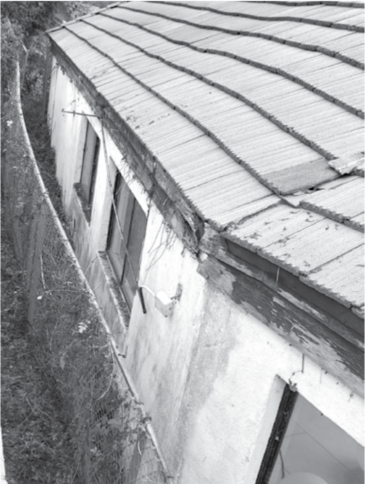
A large haphazardly built structure sits 18 inches from the neighbor's property line. The city has offered no relief.
