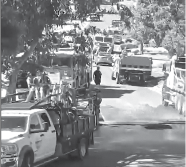
A gas line ruptured by a construction crew wreaked havoc.
