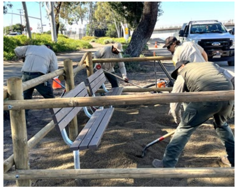
Workers from OC Parks create a rest stop along the Santa Ana River Trail.
