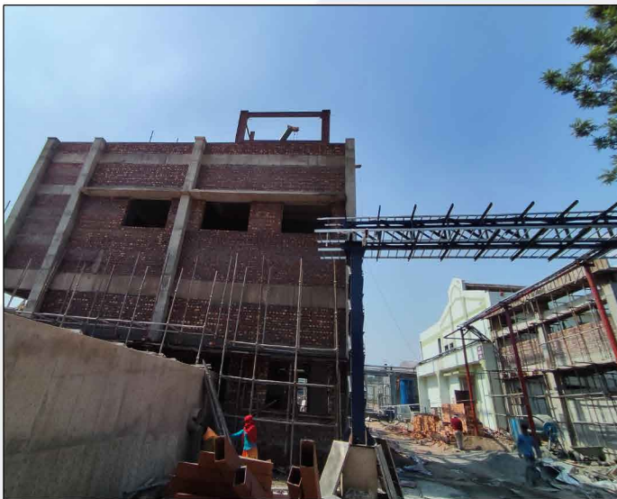
R.O. Cooling Tower
