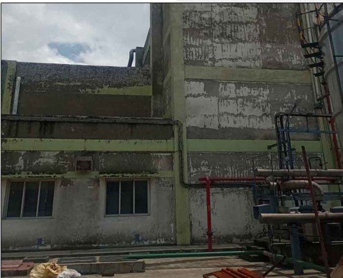
Control Building (40 TPH Boiler)
