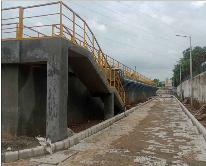
Homogeneous Tank (Periphery Road)
