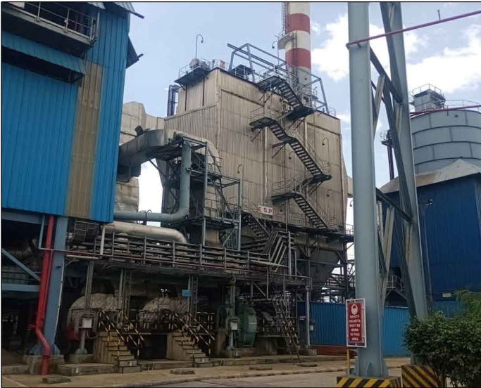
40 TPH Boiler ESP Area
