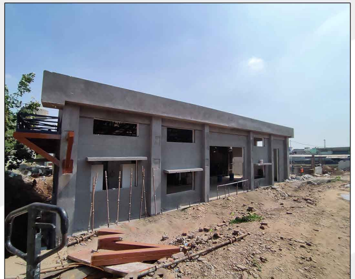
2000 MLD Under Ground R.C.C. Tank
