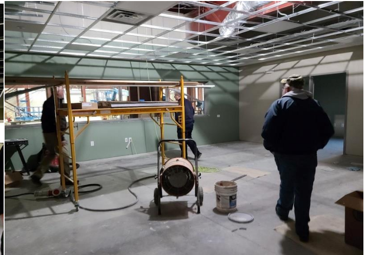
Copy Area - Windows into the Plant
