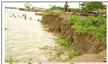
River Erosion due to Flood
