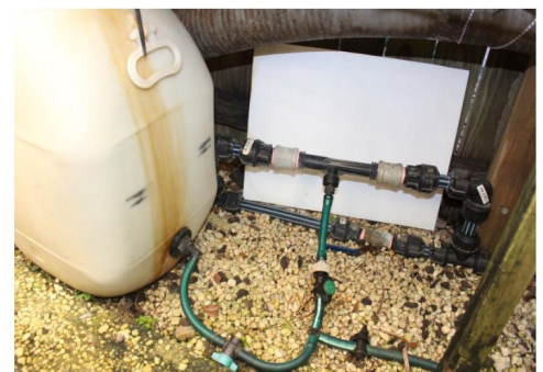
The 20 L supply tank and connections
