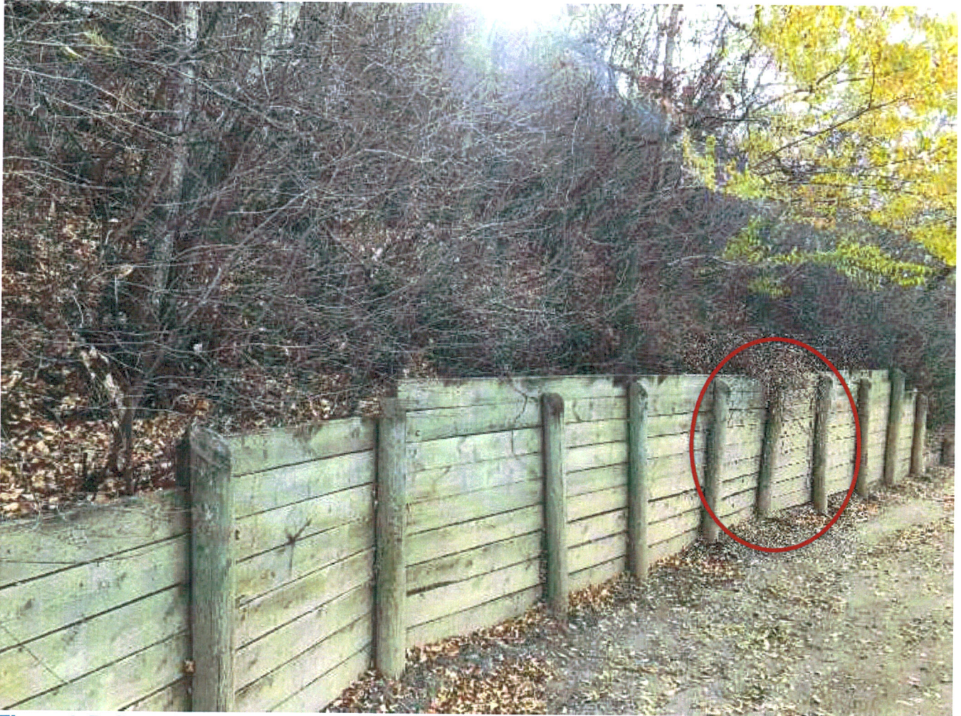
Figure 4: Deflected retaining wall, south end of Hunts Cove Crescent.
