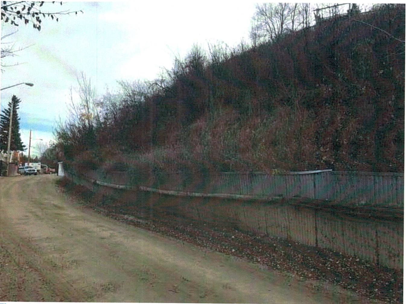
Figure 1: Failed retaining wall on Hunts Cove Crescent.
