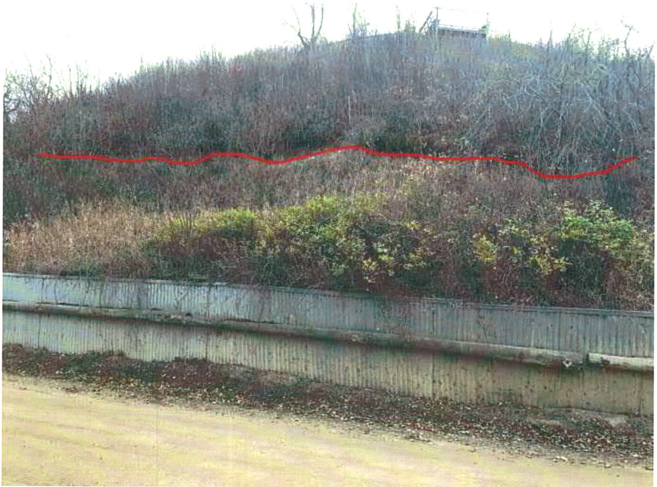
Figure 6: Slope failure above retaining wall on Hunts Cove Crescent.
