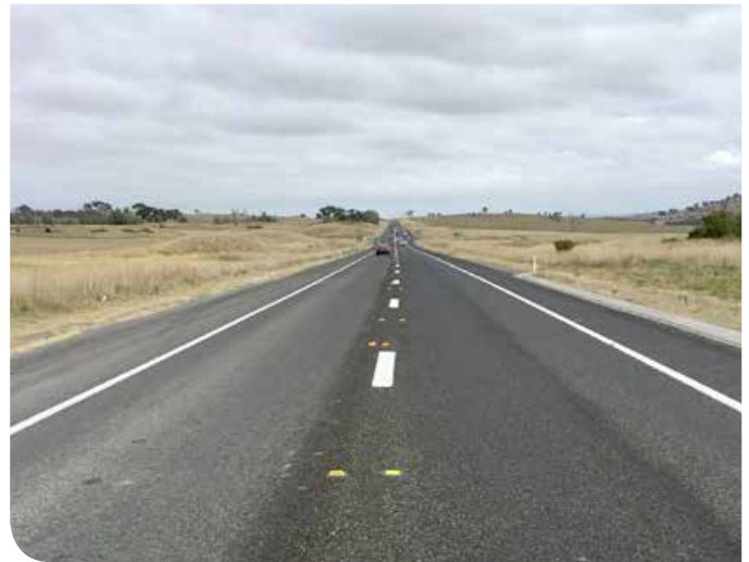
New line marking has been installed at various locations along the Barton Highway to improve safety.
