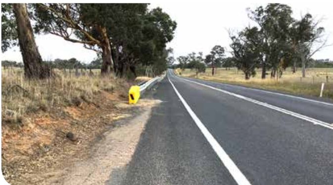
Safety barrier has been installed on the Barton Highway as part of package four work.
