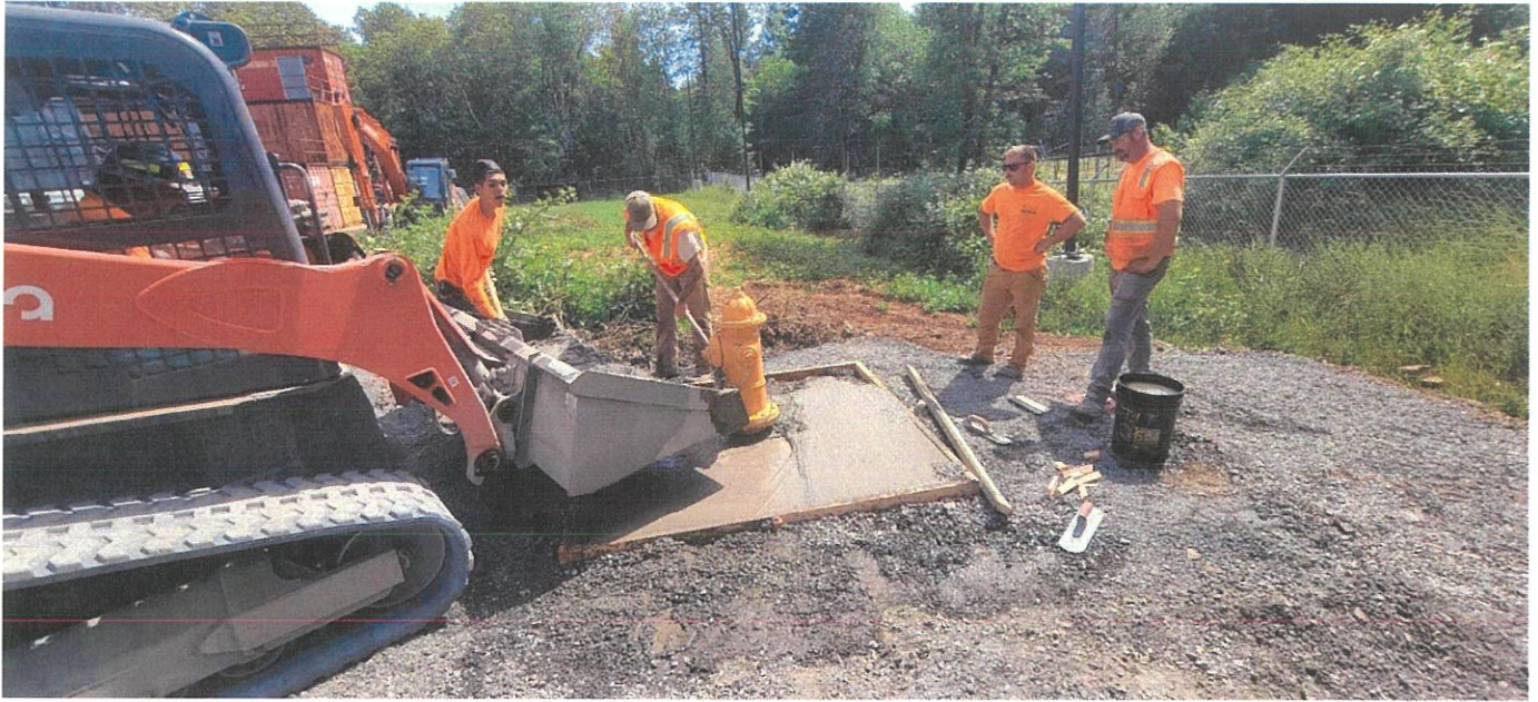
Hydrant in concrete in IVFD training area, May 20, 2026
