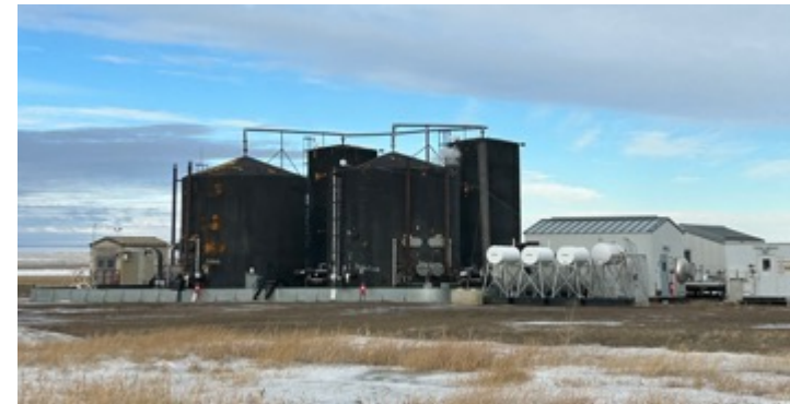
Murray Lake 7-36 main treating facility, consisting of separator, free water knockout, 5,000 bbls/d storage and water injection.
