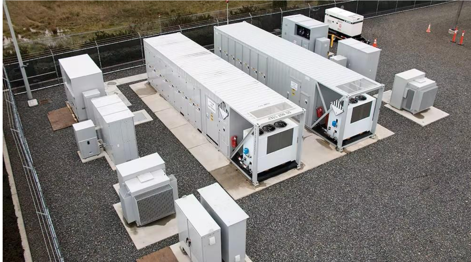
Snohomish PUD 2MW Lithium Battery Energy Storage System
