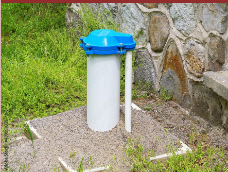
Typical above-ground portion of a domestic potable well.
