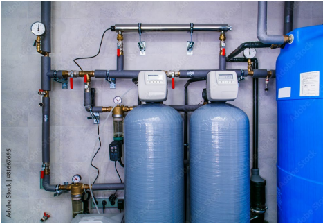
Typical residential point of entry treatment system
