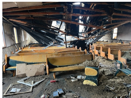
Sanctuary fire damage
