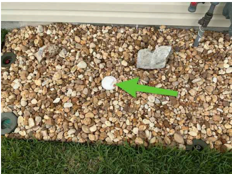
Main Drain Cleanout
