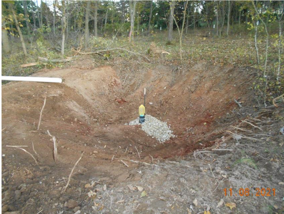
A standpipe drain would allow the trapped water to drain out via the buried culvert and prevent any additional erosion from occurring in the back of the sinkhole
