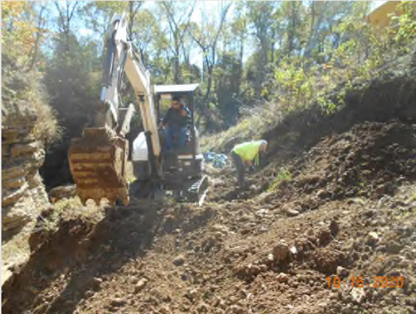
Trash, metal and tires were removed before the material was loaded onto dump trucks.
