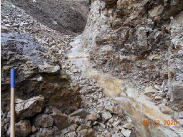
After the loose rocks were removed at the base of the hill, the water could flow smoothly.
