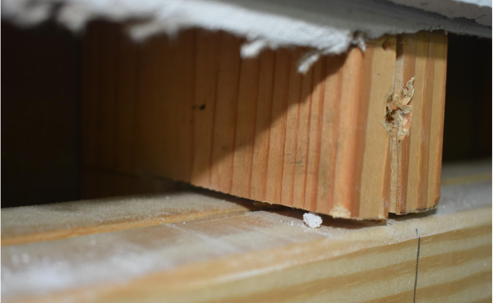
Gap issue and split stud.
