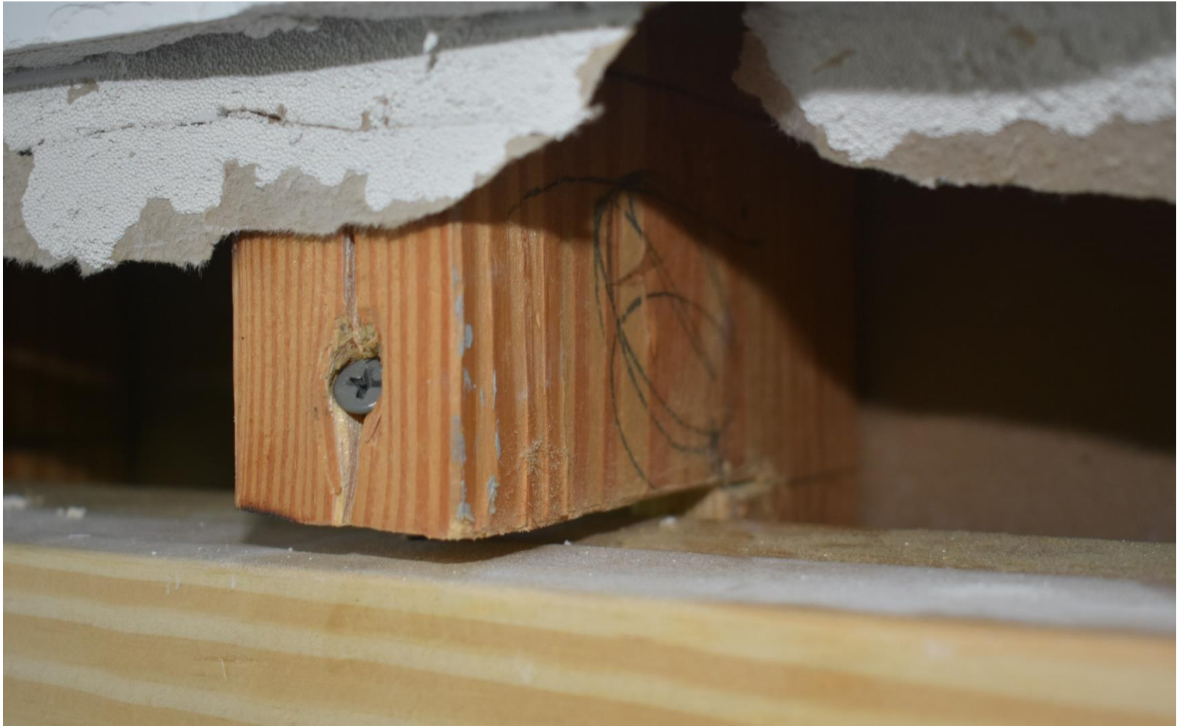
Another compromised connection between stud and header.
