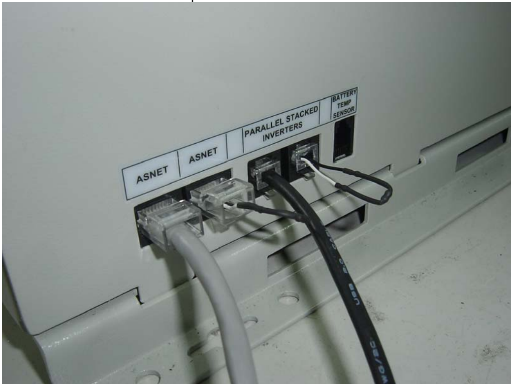
The second Inverter parallel interface and terminator resistor
