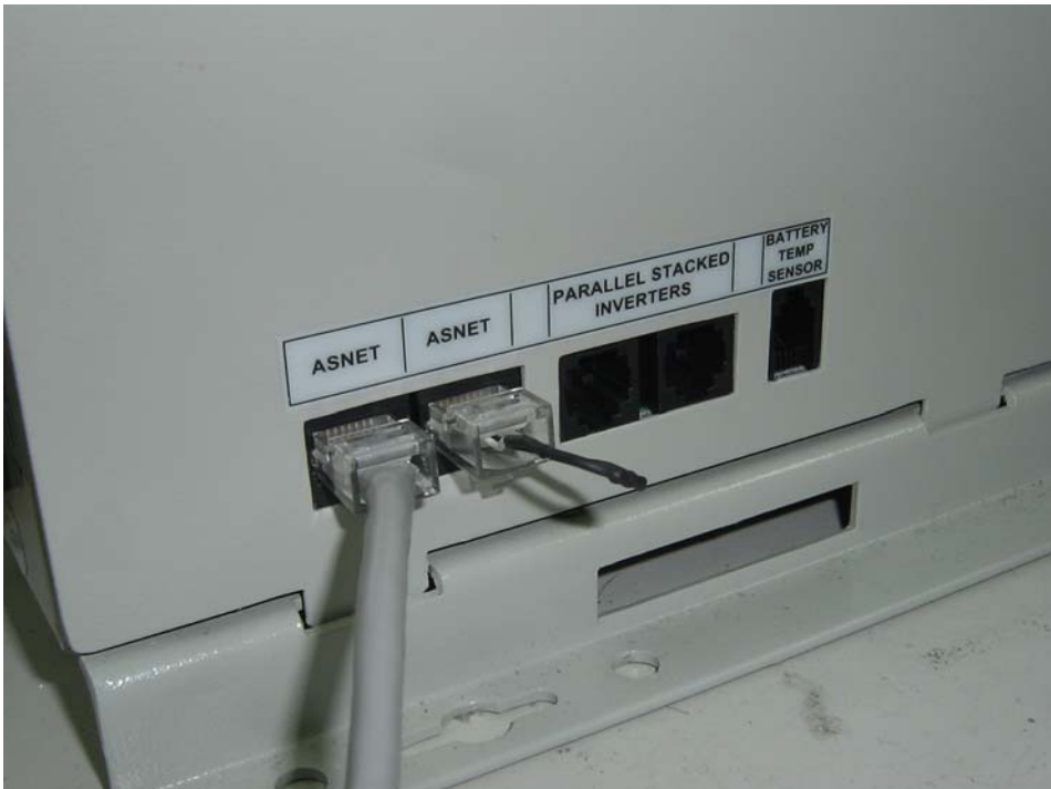
The second Inverter communication ASNET interface and terminator resistor
