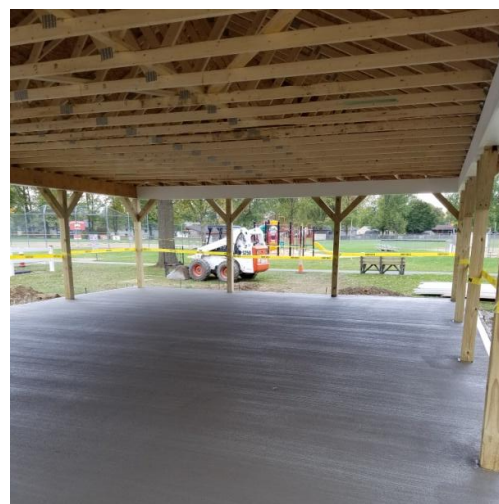
Oct. 14 th – Concrete poured, including two 10'x12' pads for picnic tables in shaded areas of the park →
