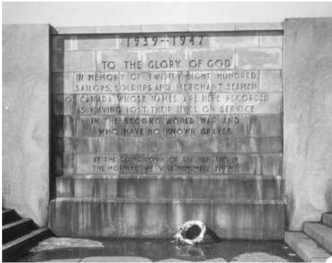
Signs of deterioration of Citadel Memorial
