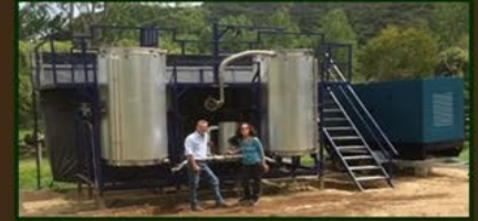
2021 - extraction plant, commissioned/ready
