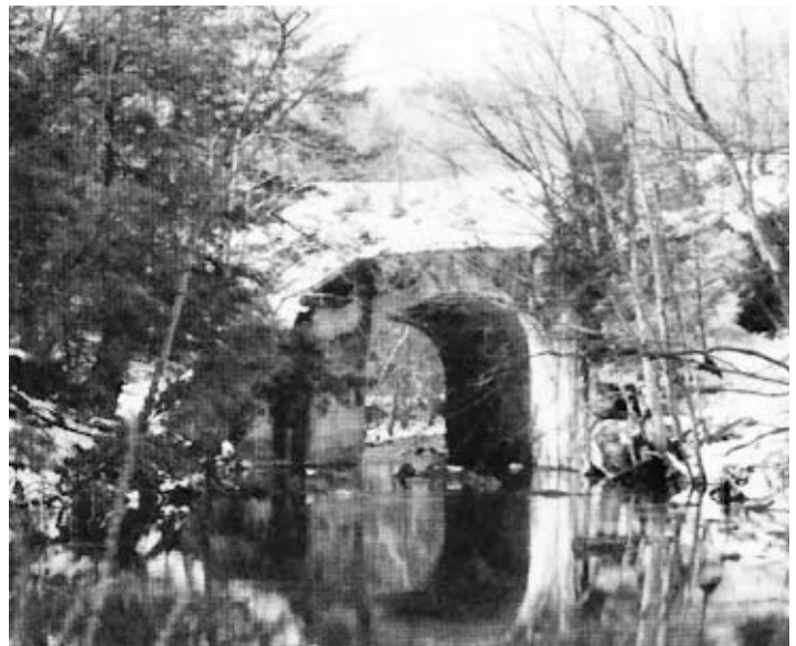
The 25-ft high concrete culvert over Shade Creek was part of the Seibert modernization program. It replaced an old wrought iron deck truss that would not withstand the heavy gannister tonnage from the GREFCO quarry.
