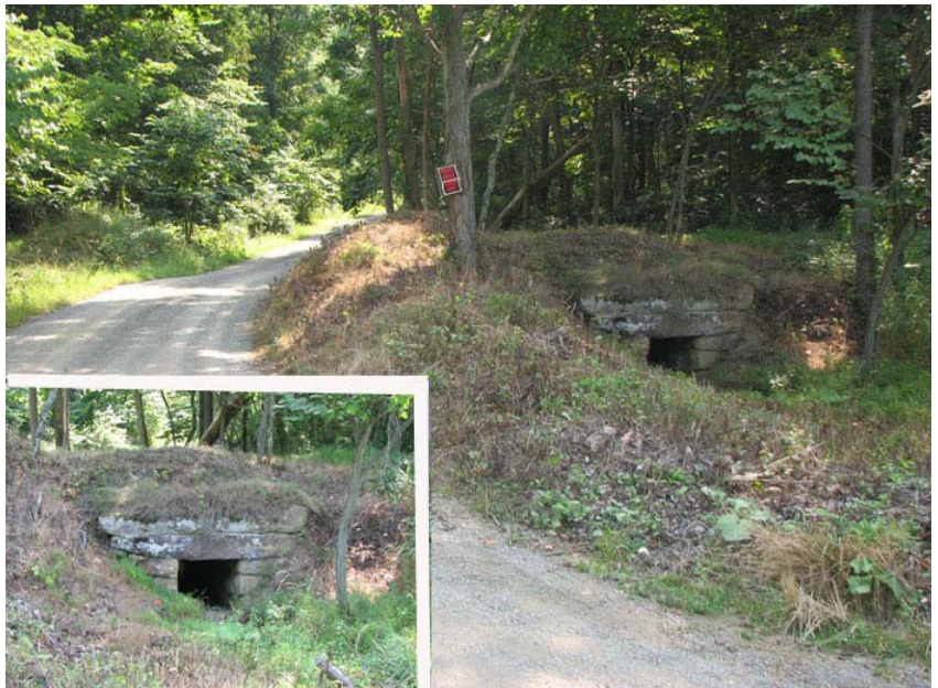
Remnants of the long-abandoned Shade Gap Branch are still visible to the trained eye. This stone box culvert just south of the grade crossing over Shade Valley Lane near the Cedar Rock station is one example. Vagel Keller photo, 2009
