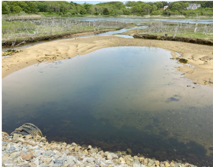
Figure 3 — Upstream Culvert Outlet, Scour hole and Shoaled Sediment (facing east)
