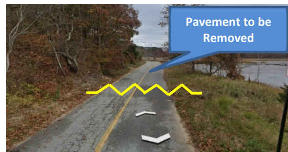
Figure 10 — Limit of Pavement Removal South of Mill Pond Road / Depot Road Intersection (facing south)
