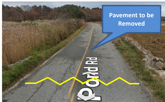
Figure 13 — Approximate Limit of Pavement Removal and Channel Breach South of Mill Pond Culvert (facing south)
