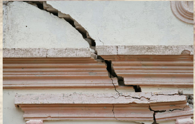
Watch for damaged buildings and falling debris
