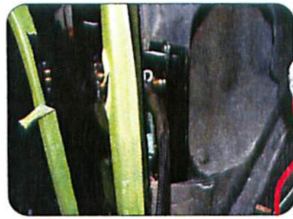
The Classic Industries electronic instrument controller is mounted in the driver's side kick panel to free up space under the dash.
