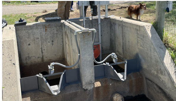
New meter system from ditches
