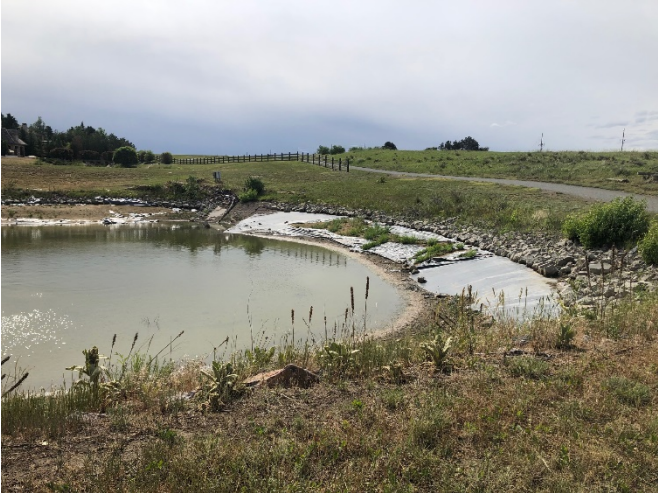
Liner ripped starting condition, Pond 8 one-third full
